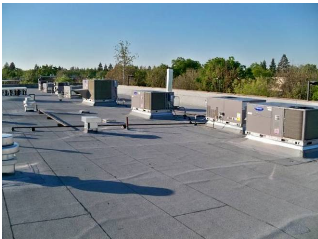
5. View of HVAC package units on Building 1445 roof (typical of most buildings).
