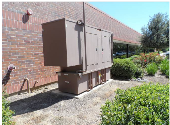
6. View southeast of standby generator and diesel fuel "belly" tank at northwest corner of Building 1445.
