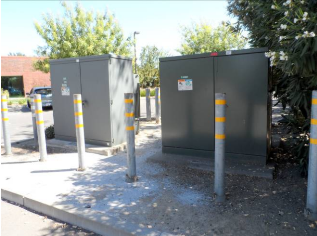
19. View southeast of PG&E transformers in central portion of subject property (typical).
